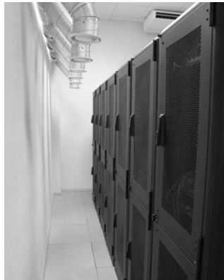
Figure 1. Back side of racks
